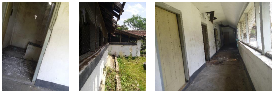
Figure 8. Building decay of first house.
