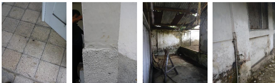
Figure 11. Building decay of second house.
