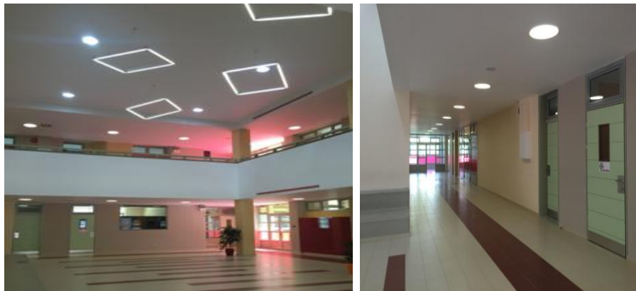
Figure 10. Lightway sun tunnels installed in main entrance and corridors
